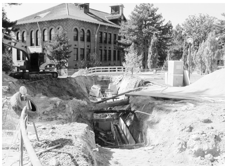
The real crater from the water line break. The picture on the front is the Kennecott Copper Mine.
